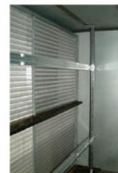
Fig 8 Horizontal Lamp Placement for Coil Surface Disinfection
