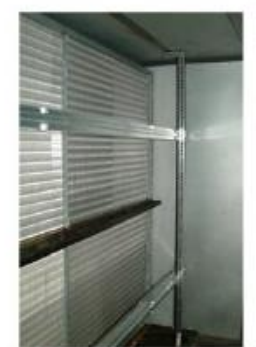
Fig 8 Horizontal Lamp Placement for Coil Surface Disinfection
